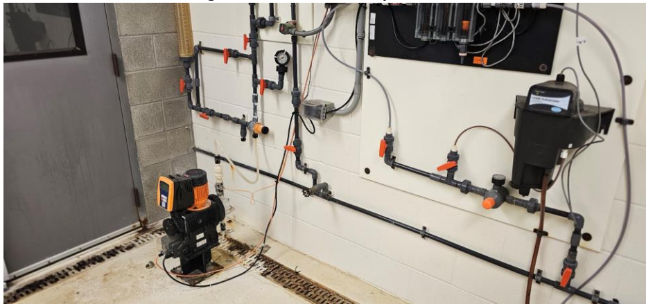
Figure III-4: Chlorination Unit with Corrossion Evident
