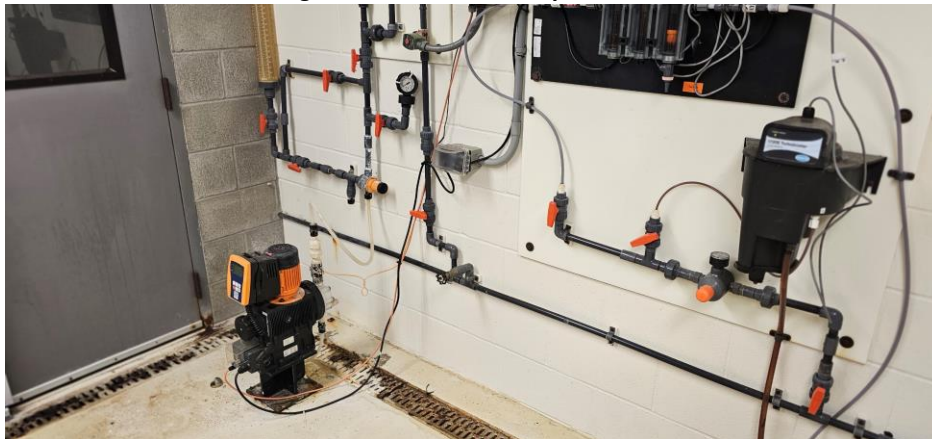
Figure III-4: Chlorination Unit with Corrossion Evident
